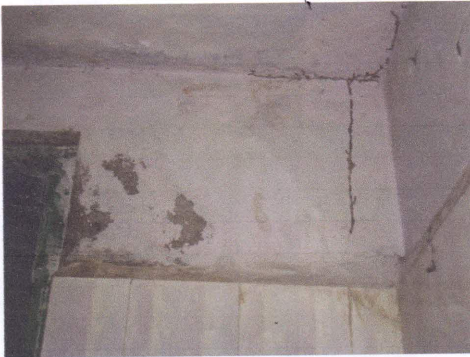
Moist surfaces and chipping off plaster in the toilet.
